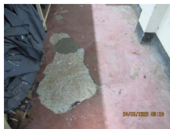
Uneven and broken floor observed on production floor located on ground floor of shed no.1. (2).JPG
