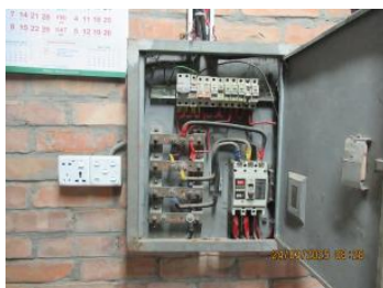
Electric ebonite sheet was missing for electrical distribution board..JPG
