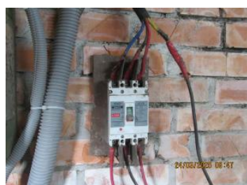
Loose and multi electrical wire connection found in the facility. (2).JPG
